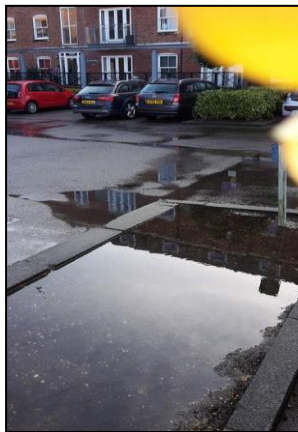
SE corner of NM4/5 footprint flooding into the road
